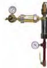
Fuel Gas Station Drop
