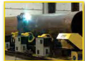
Ready for fit up and/or automated welding, then index for next section to be added
